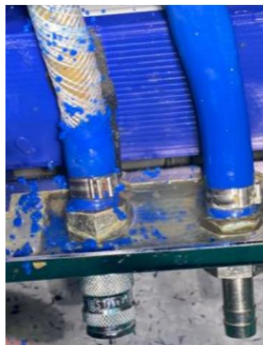
Figure 2: Degraded vs. intact blue colored hose
