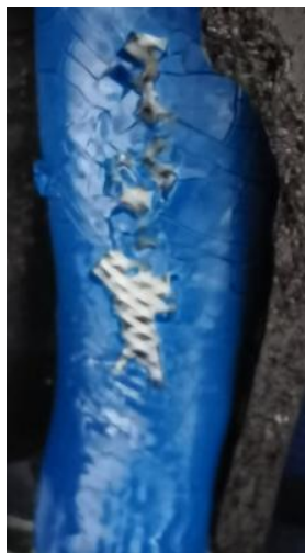
Figure 1: Degraded drain hose
