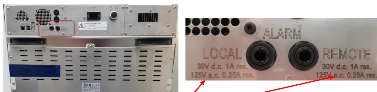
Alarm Connectors labelling
